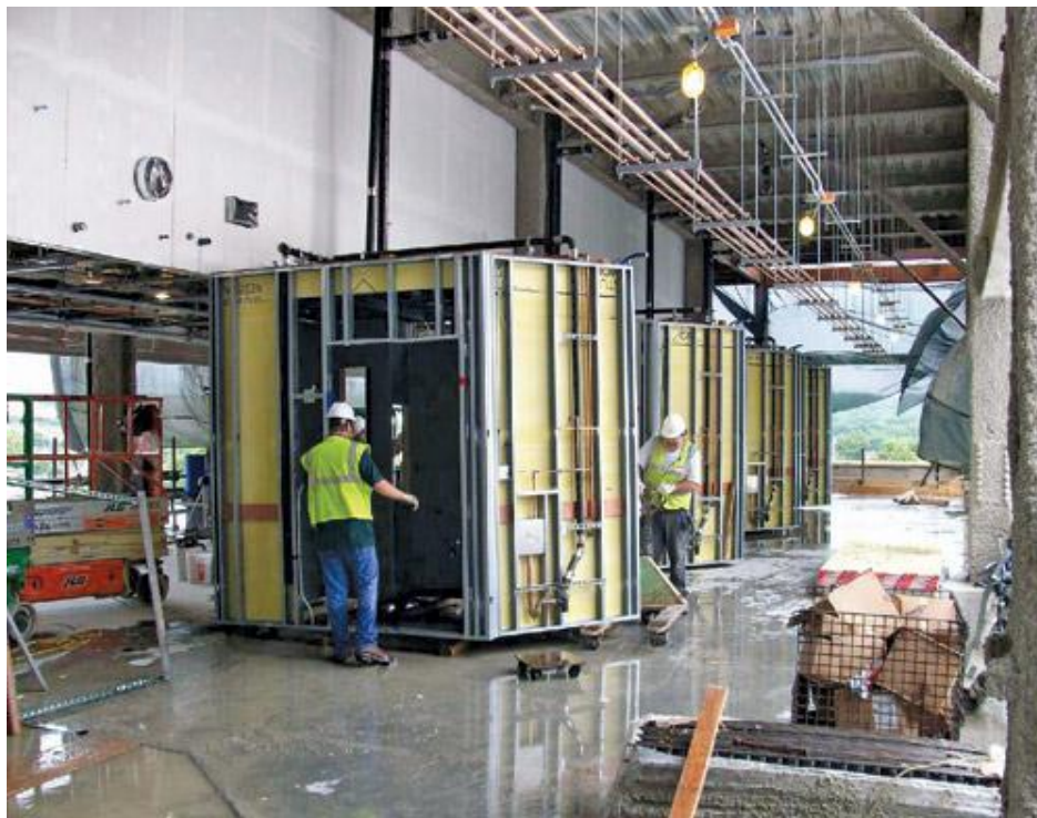
Figure 2-1 Shows the pre-fabricated module under construction for the Miami Valley Hospital in Dayton, Ohio (Post, 2010)
